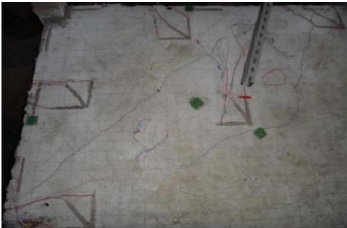
(a) Experimental Cracks of Slab (P1) [20]
