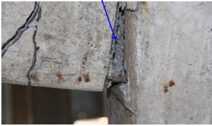
(a) Experimental Cracks at the Longitudinal Beam [21]
